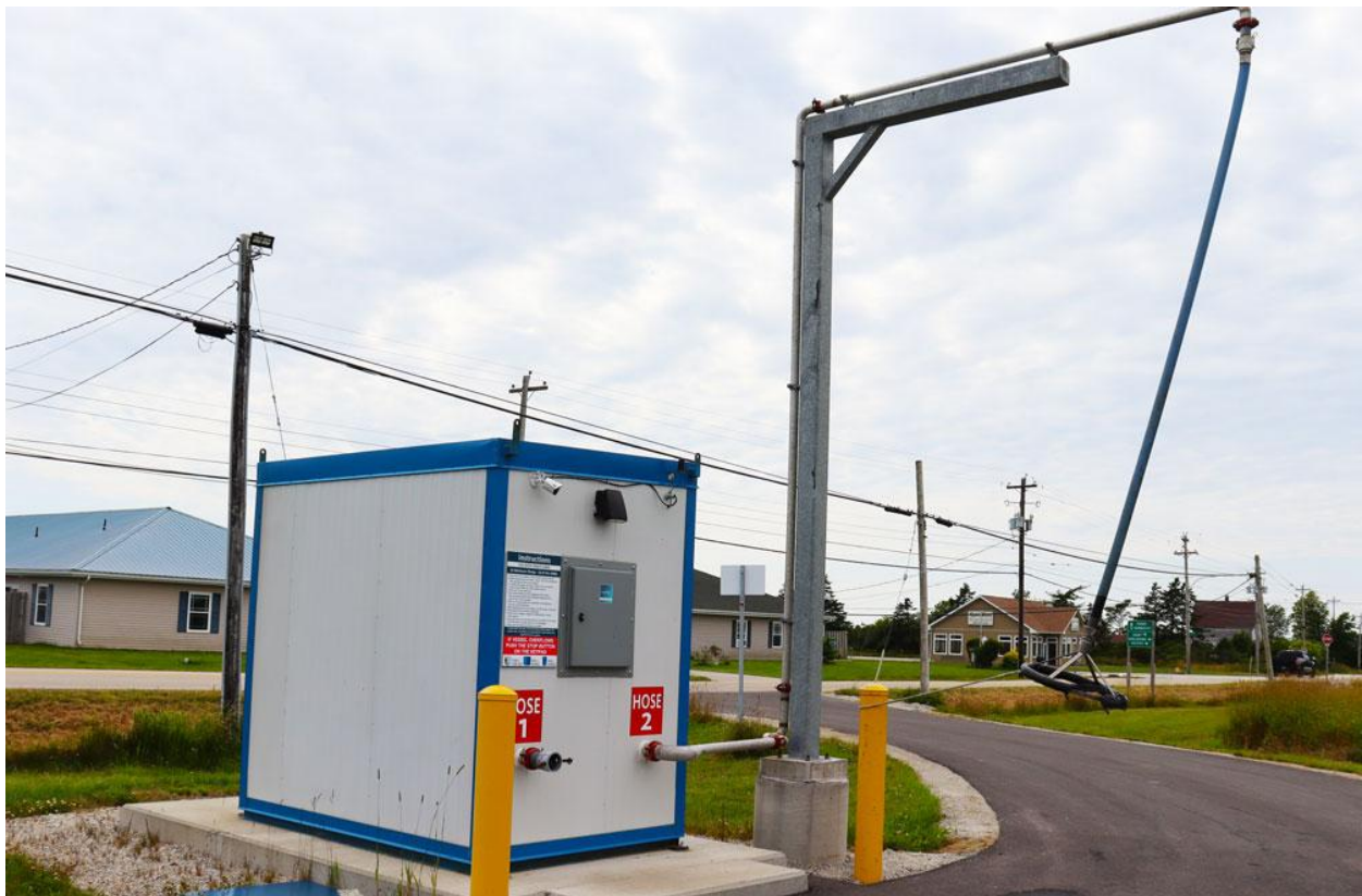
Figure 21: Bulk Water Station in the Town of Yarmouth.
